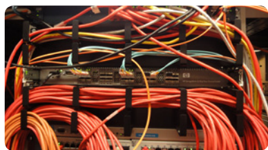
Each 12big Rack Fibre array is connected to HP SAN Fibre Channel Switches via their dual fibre channel host ports. Two host ports guarantee optimal performance and redundancy in case one should fail.
